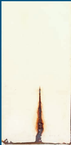
One coat of Series 91-H 2 O Hydro-Zinc, then two coats of two-component epoxy
