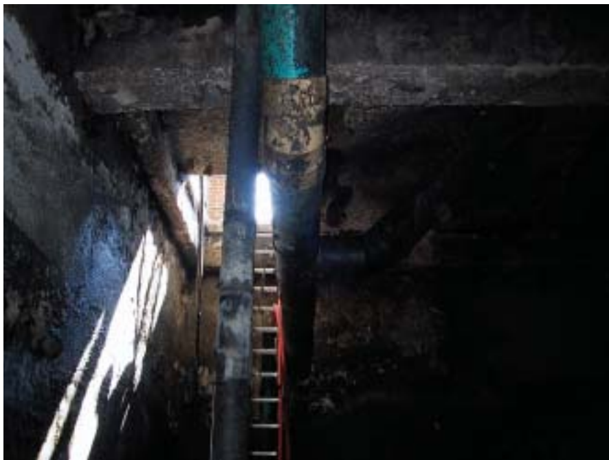
Deterioration of concrete sludge holding tank after 10 years of H 2 S corrosion.
