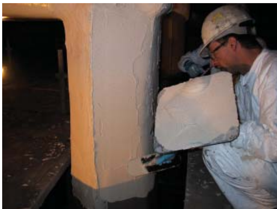
Trowel application at 125 mils of 100% solids epoxy mortar system designed for elevated H 2 S permeation.
